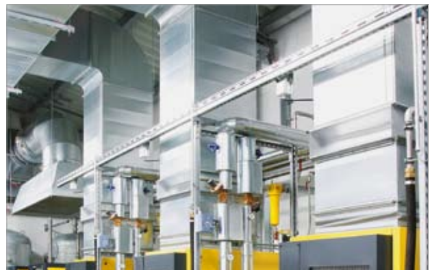
Ducting for heating of adjacent rooms
