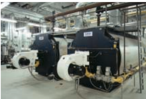
UNIMAT Heating Boilers in a public facility:
