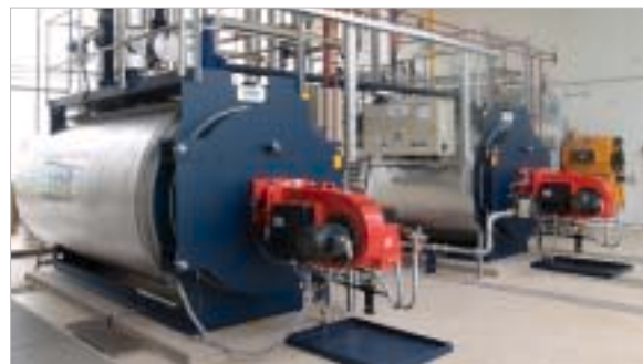
Two type UT-M UNIMAT hot water boilers in a packaging plant to supply heat to the halls
