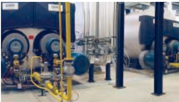
Two type UT-HZ UNIMAT hot water boilers in an airport, supplying hot water and heating
