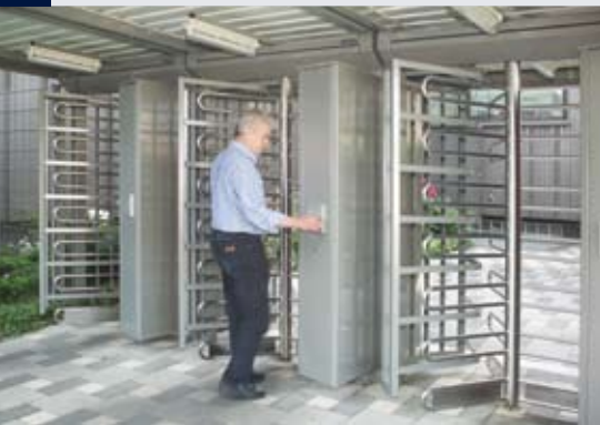
As staff access: multiple unit installed in the fence surrounding the plant
