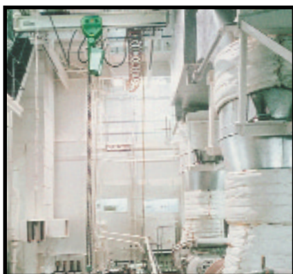
ENGINE ROOM OF A SHIP
