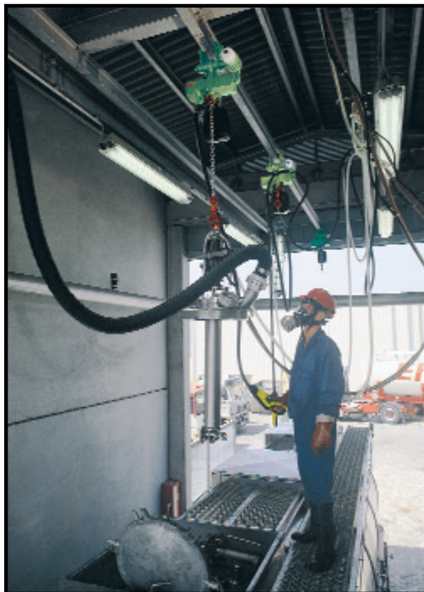
TANK CLEANING PLANT
