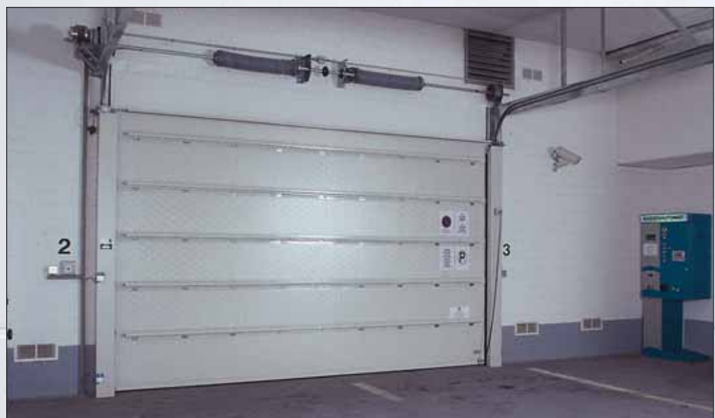
T30 Sectionaltor in Tiefgarage.
